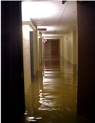
3-feet of water throughout the halls and Archive
